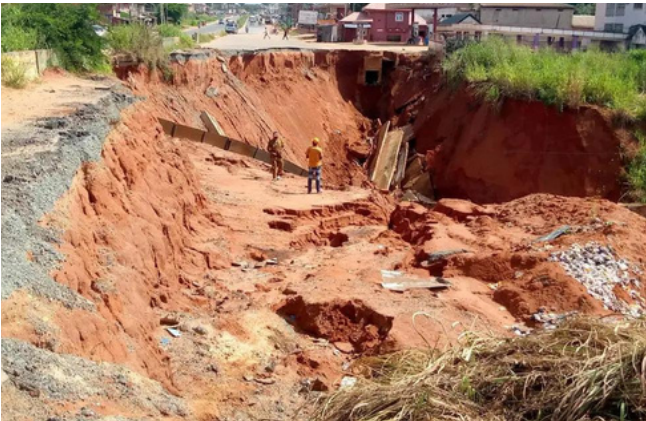
Deep erosion in Ogwashi-Uku community, Delta State
